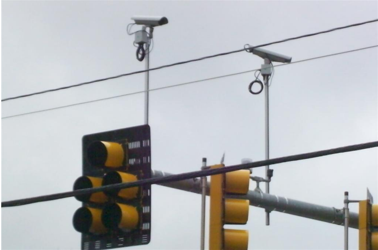
Photo of new video vehicle detection devices installed on new traffic signal systems.
