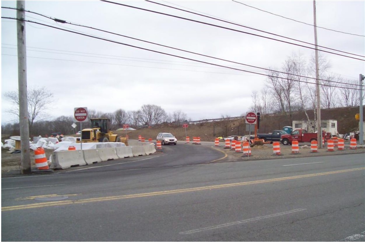
View of new off ramp from Route 128 North to Route 62 recently opened for eastbound movements.
